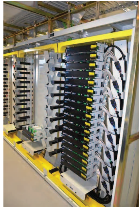
Exhibit 9-6: Example of Cabinet Install
